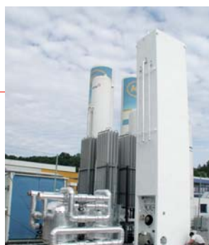
Messer's newly-designed on-site plant
