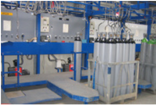
Filling station for ultra-purity gases
