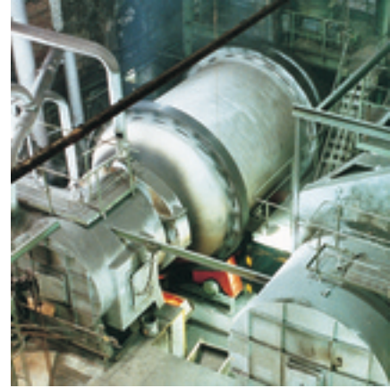
Hazardous waste incineration: Rotary furnaces can swallow almost anything – and do so more efficiently
