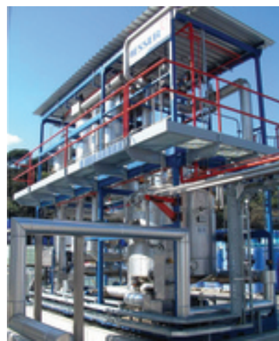
Solvent recovery with Cryosolv®
