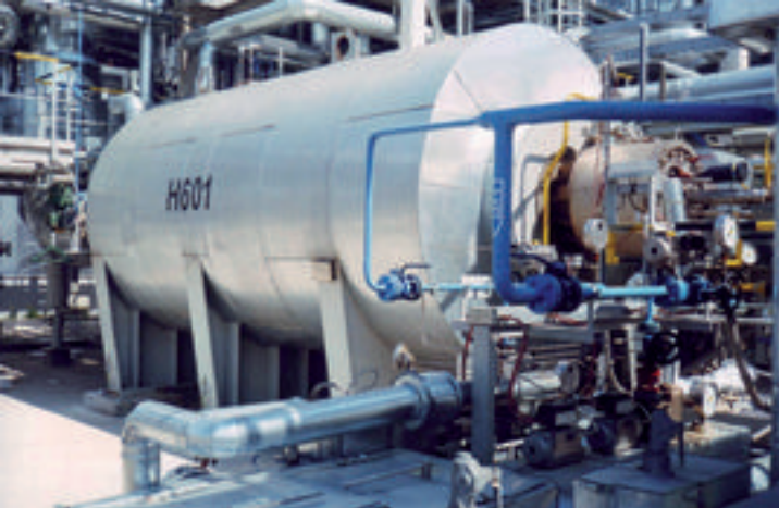
A targeted O 2 supply increases the efficiency of cracking units.
