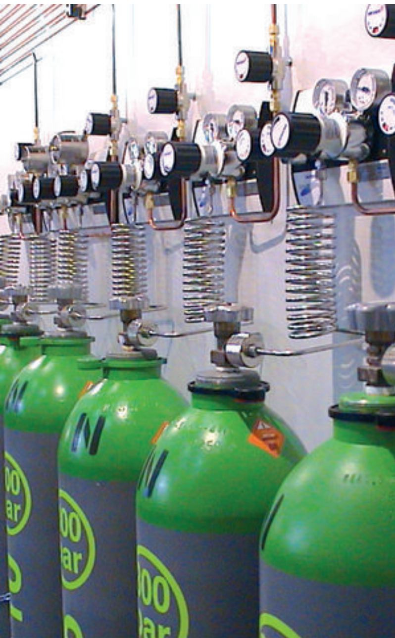
Central gas supply - gases on tap
