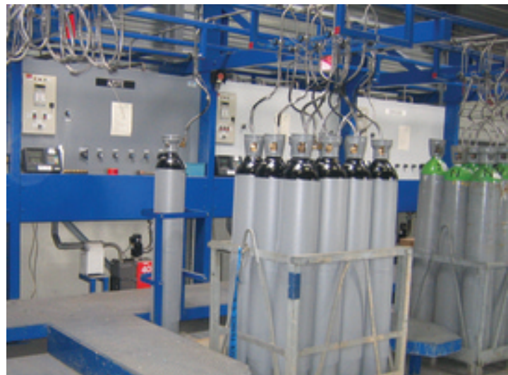
Filling station for high-purity gases
