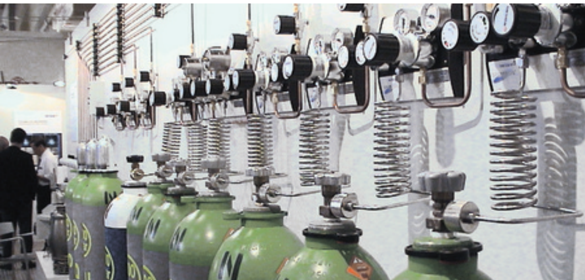
Central gas supply - the safe solution
