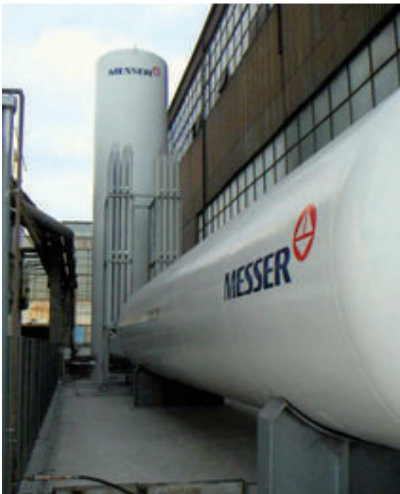
Figure 9: Storage vessel for liquid nitrogen (standing) and gaseous hydrogen (horizontal)
