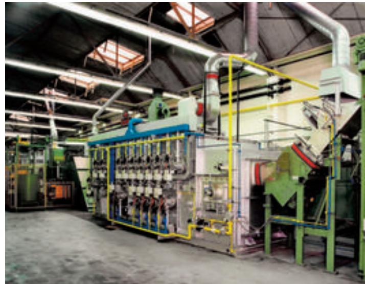
Fig. 4: Continuously conveyor furnace from Aichelin
